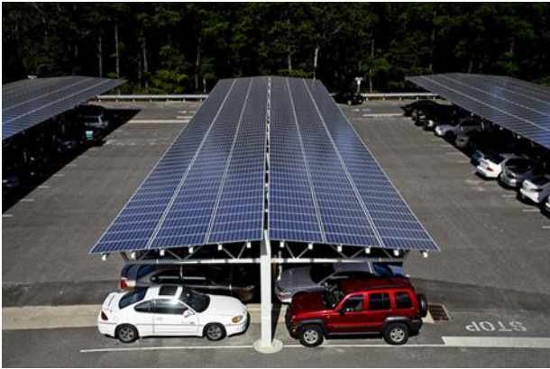
Figure 4-8 Carpark Shade Structure Mounted Solar Panels Angled East-West
